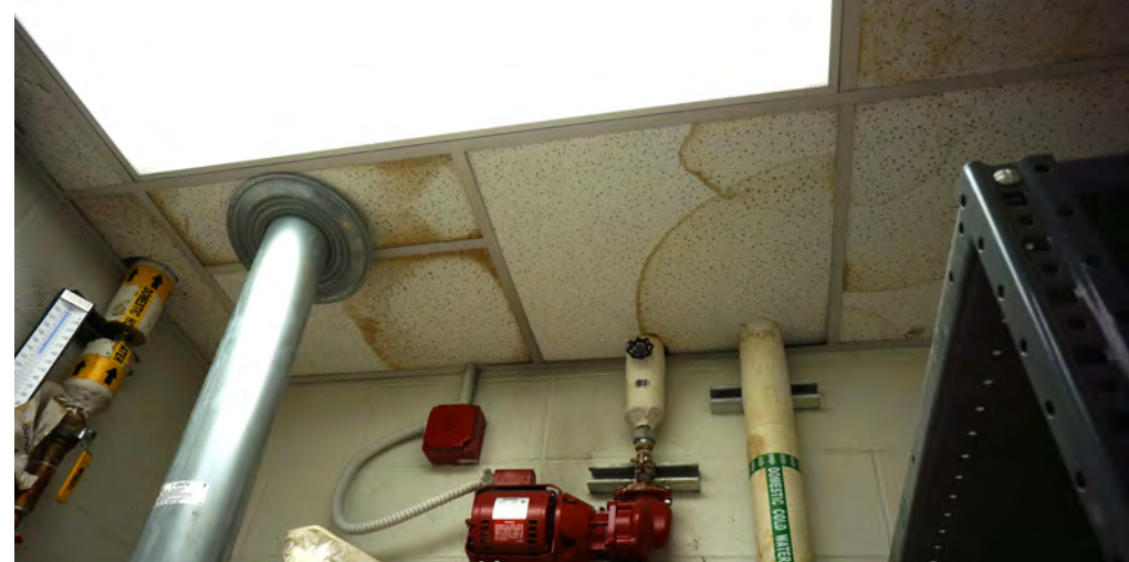
Roof leakage was a common occurrence around the Fire Station, including in the break room, offices, and over electrical equipment.
