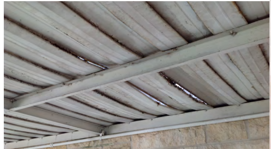
The canopy around the Golf Course Club House has experienced so much weathering that it is severely deteriorating and damaged, causing it to warp and fall down in some places.
