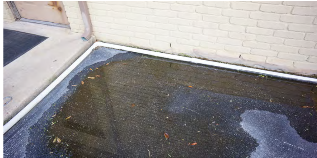
This photo shows the water left from a rain storm at the City Maintenance Staff Building. This illustrates the lack of drainage on the site.
