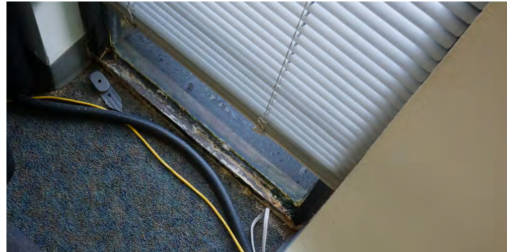
This window is an example of a number of windows in the building that are not sealed properly and causing water leaks and corrosion.
