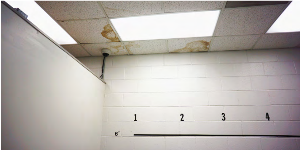
The ceiling in the Police Station’s Lineup Room shows signs of water damage from high humidity and water leaking.
